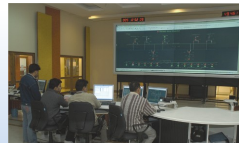
SCADA Control Centre at Kalkaji, Delhi
