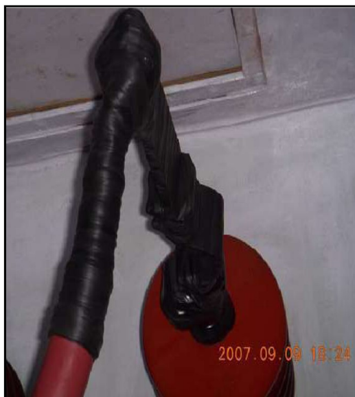
Application of EPR tape (3M-Scotch-130C)
